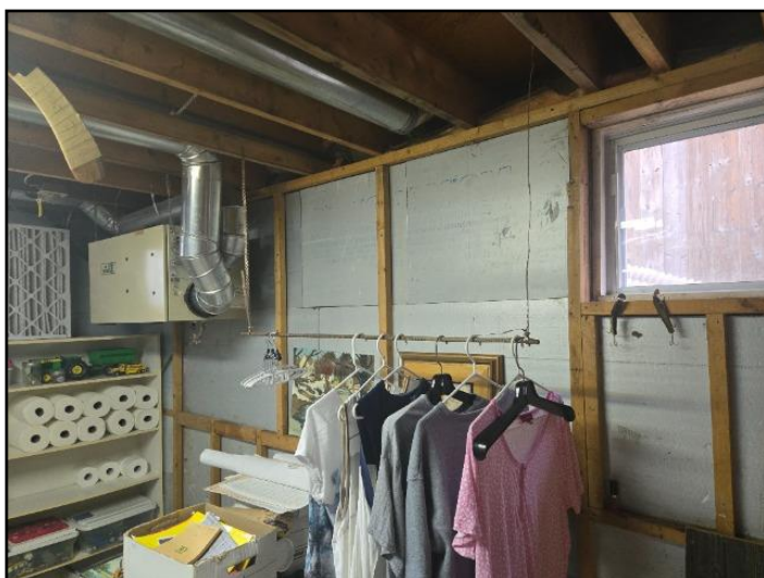
Exposed combustible insulation
