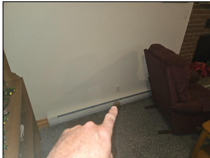
Electrical receptacle above heater
