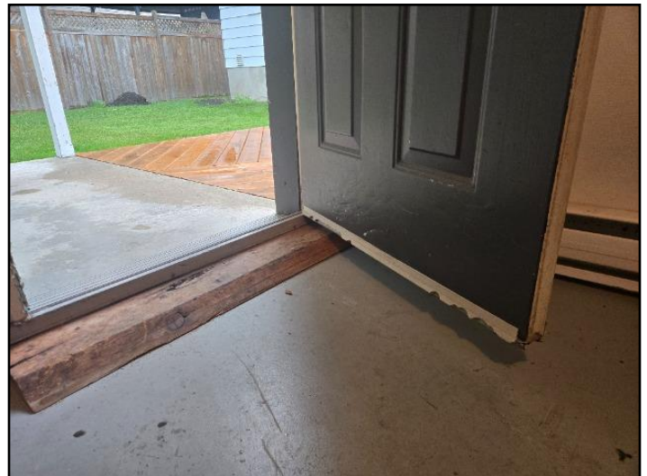
Shed Weatherstripping ineffective
