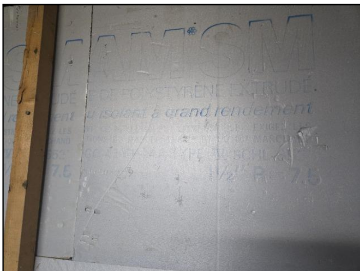
Exposed combustible insulation
