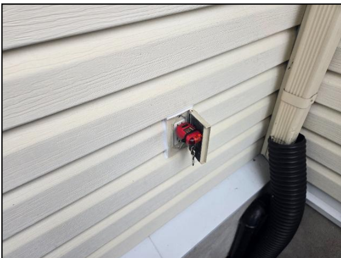
Test faulty on GFCI
