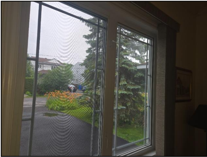
Failed window seal
