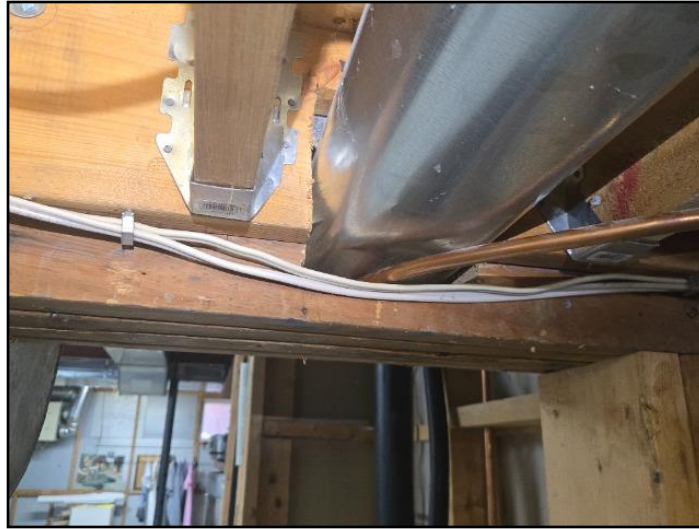
Wood header compromised
