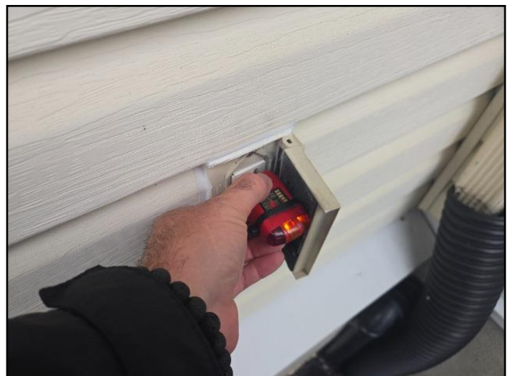
Test faulty on GFCI
