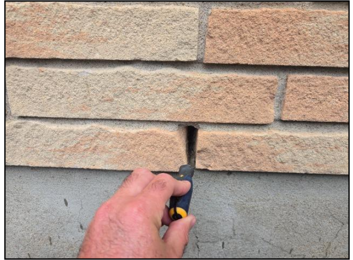
Weep holes - obstructed
