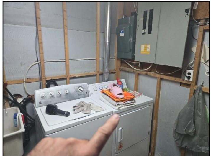
Box location poor
