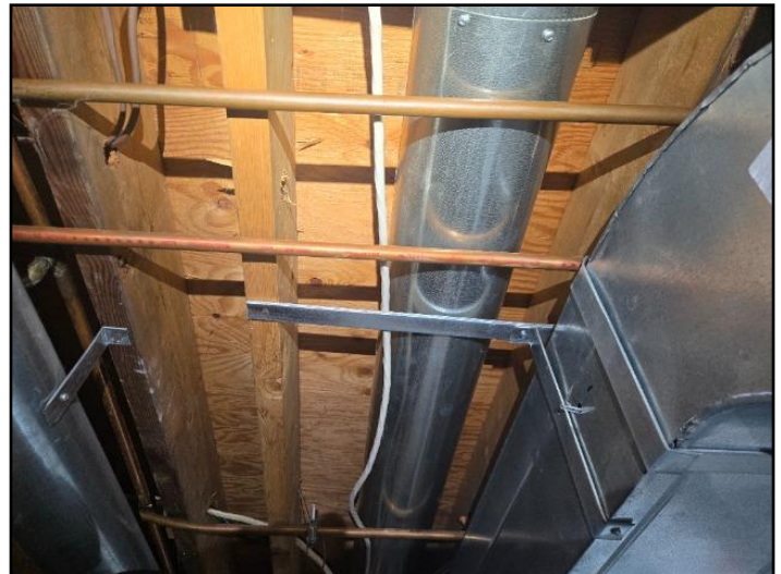
Isolated from the metal ductwork
