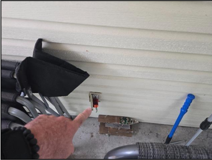
Test faulty on GFCI
