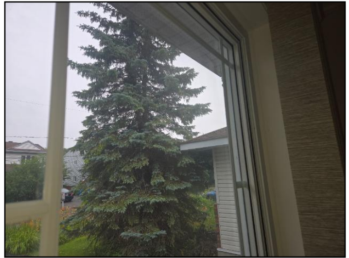
Failed window seal
