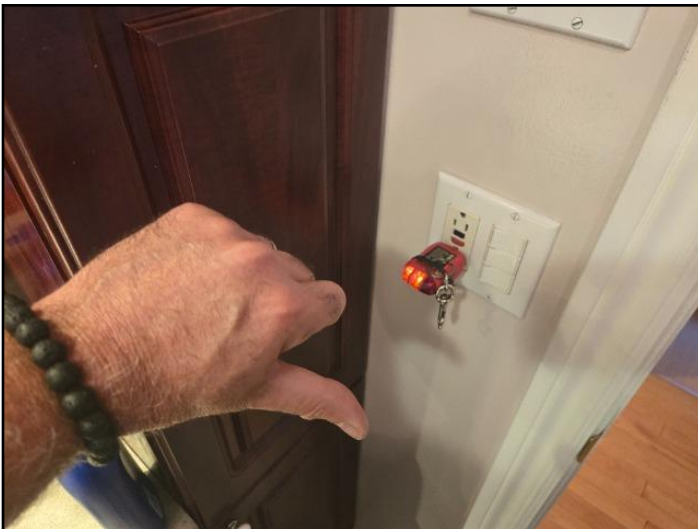
Test faulty on GFCI
