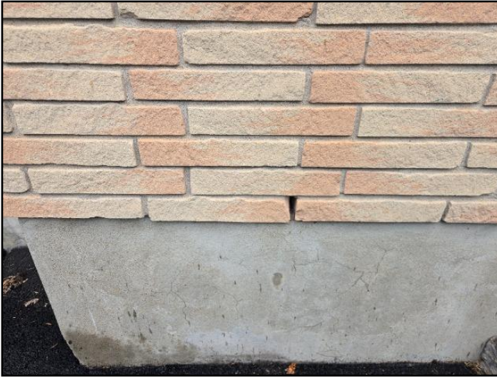
Weep holes - obstructed
