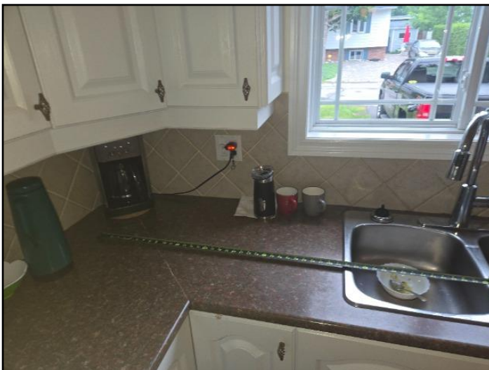
No GFCI/GFI (Ground Fault Circuit...
