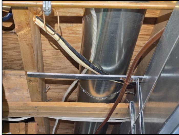
Wiring touching heating supply ductwork
