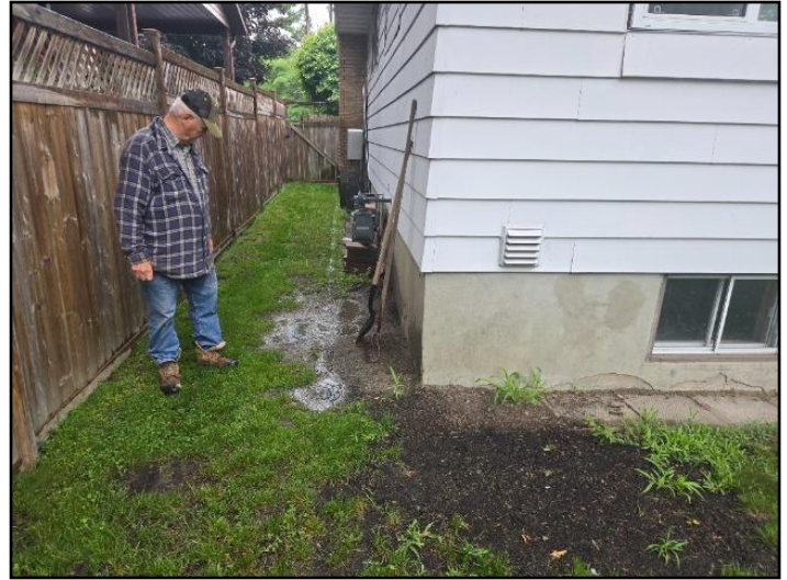
Improper slope or drainage
