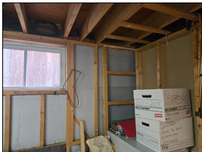
Exposed combustible insulation
