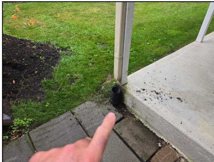
Discharge below grade
