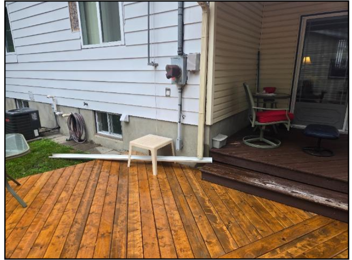
Discharge too close to building
