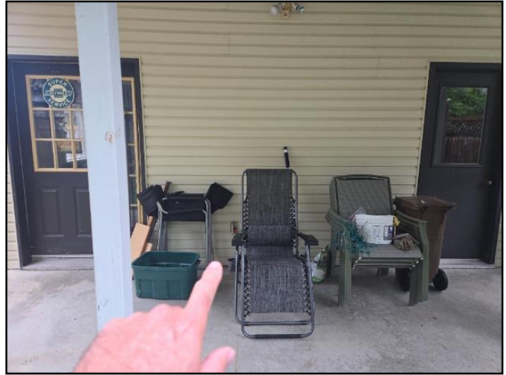
Test faulty on GFCI
