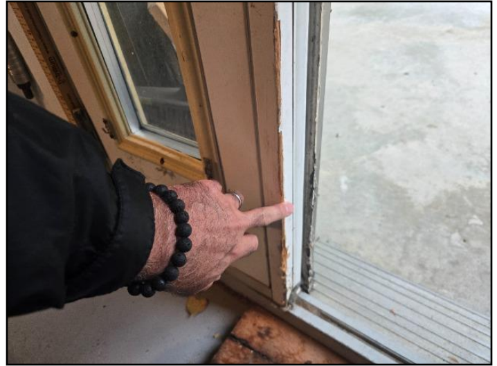
Shed Weatherstripping ineffective
