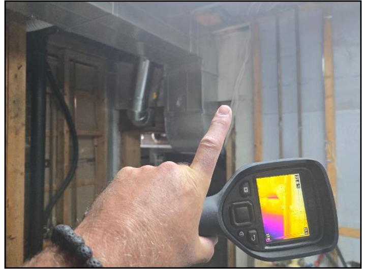
Location of minor crack
