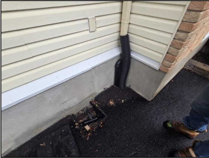
Discharge below grade
