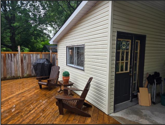
Shed Weatherstripping ineffective
