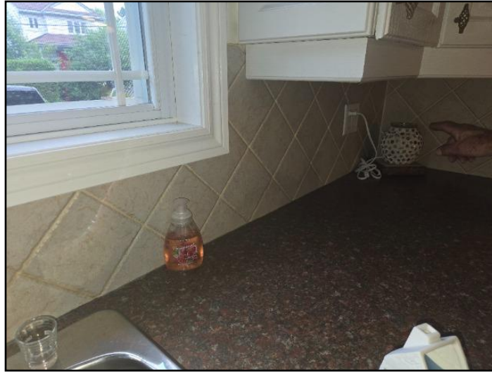
No GFCI/GFI (Ground Fault Circuit...
