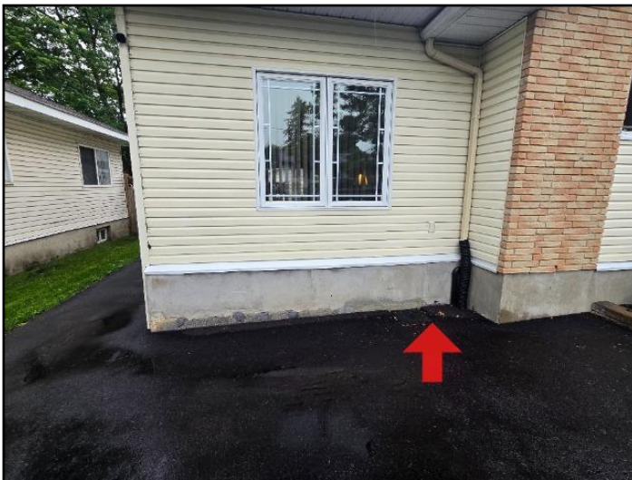
Sump location interior
