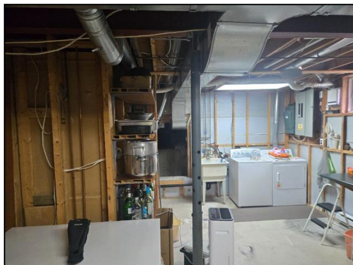
Exposed combustible insulation
