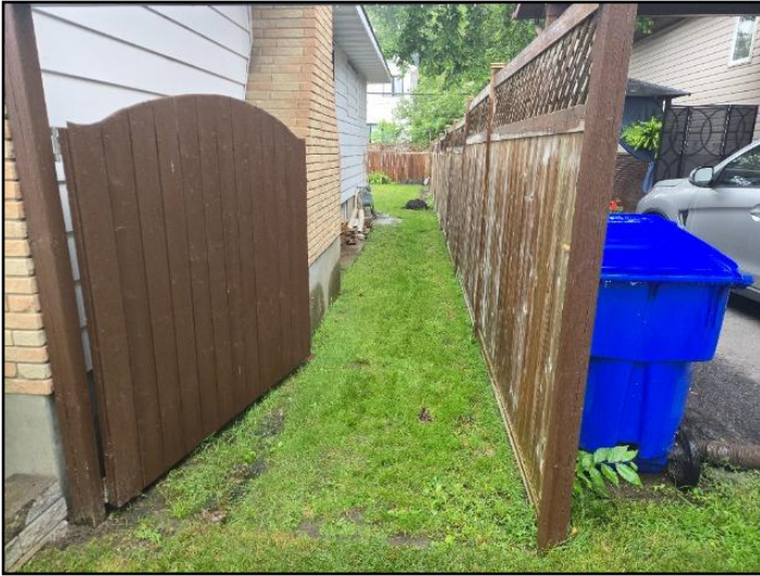
Improper slope or drainage
