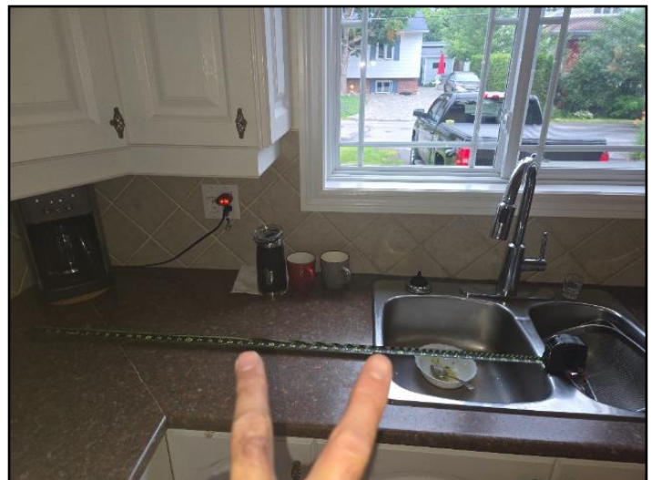
No GFCI/GFI (Ground Fault Circuit...
