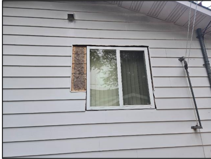
Exterior siding incomplete
