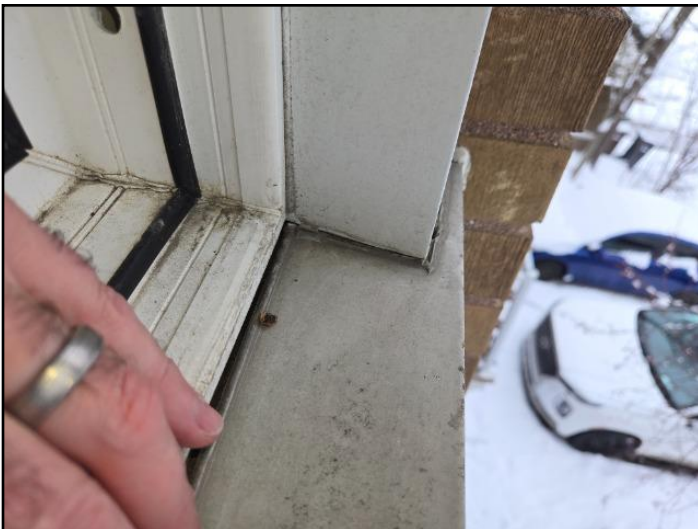
Caulking missing or ineffective
