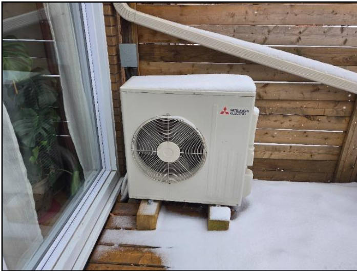
Heat Pump Outdoor Unit
