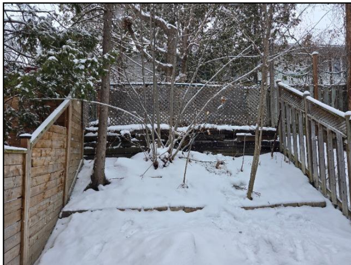
Wall exhibit signs of deterioration
