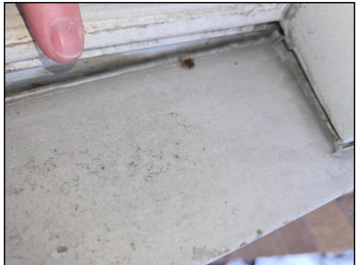
Caulking missing or ineffective
