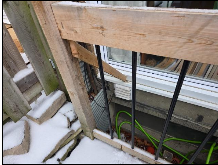
Openings between spindles (balusters) too...
