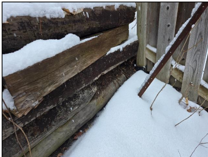
Wall exhibit signs of deterioration
