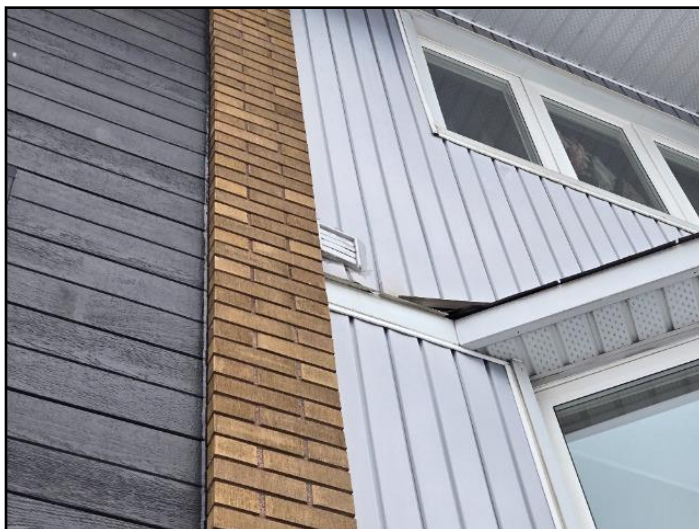
Improper Plastic Vent Termination
