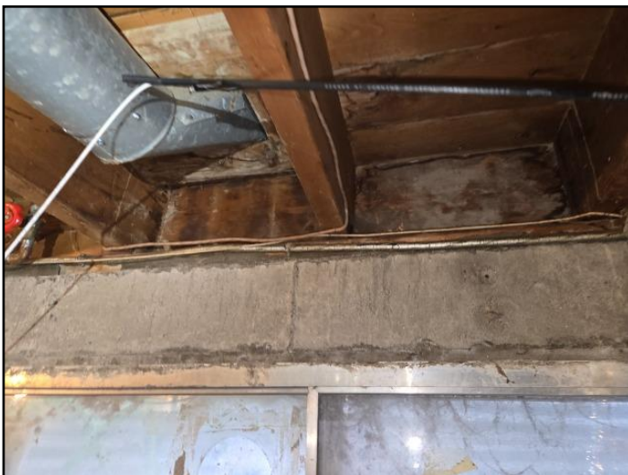
Missing at rim joist
