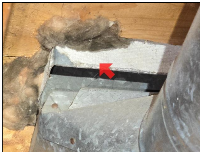
Suspected asbestos-containing material (ACM)
