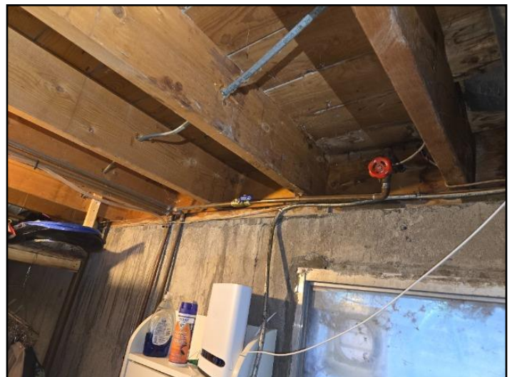
Missing at rim joist
