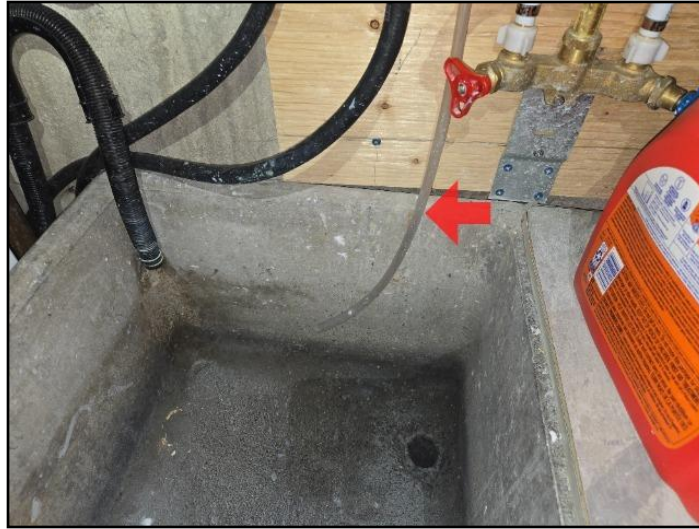
Improper discharge point
