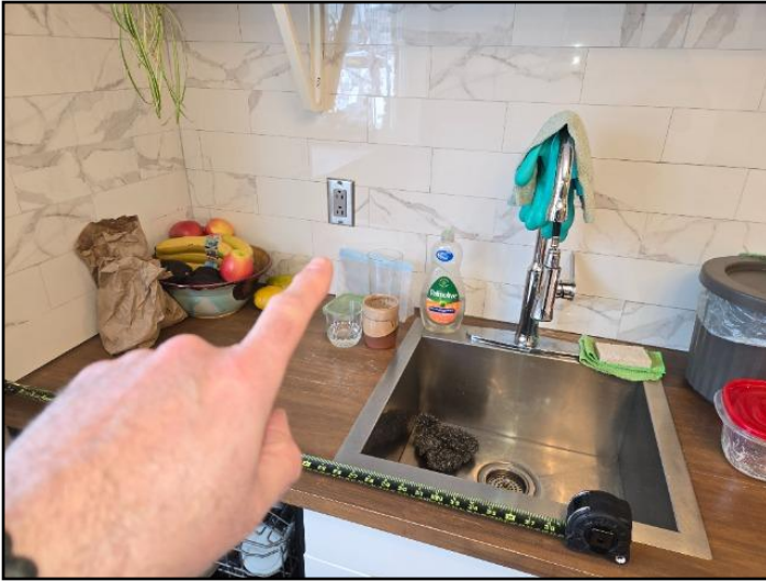
No GFCI/GFI (Ground Fault Circuit...
