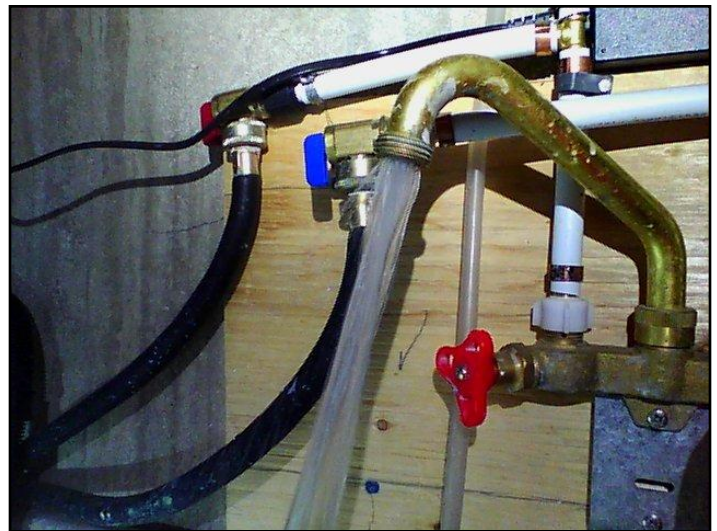
Water too hot
