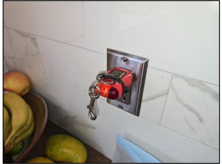
No GFCI/GFI (Ground Fault Circuit...
