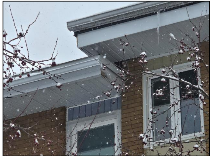
Loose or missing pieces
