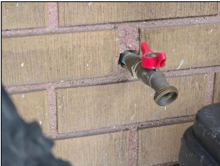
Caulking missing or ineffective
