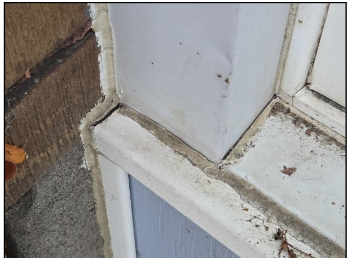
Caulking missing or ineffective
