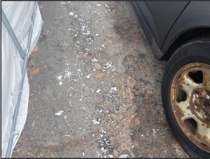
Cracked or damaged surfaces
