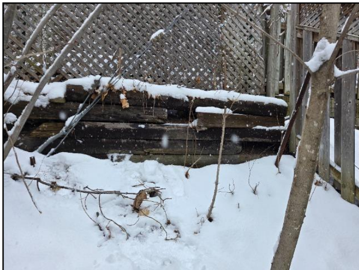
Wall exhibit signs of deterioration
