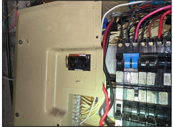
Wires crossing bus bar
