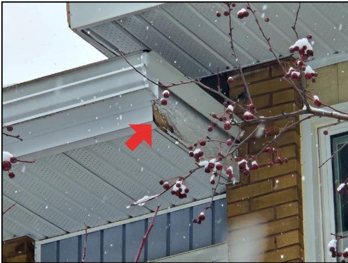
Loose or missing pieces
