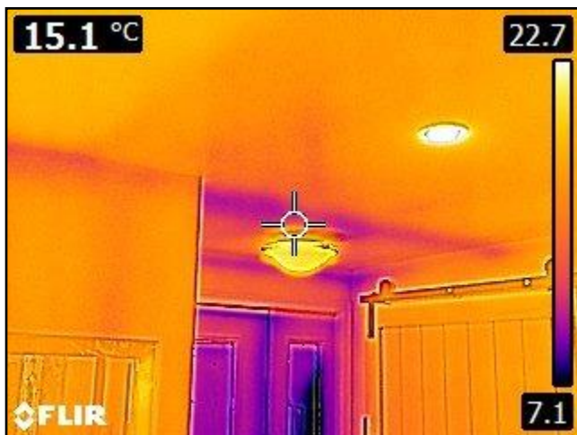
Gaps or voids
