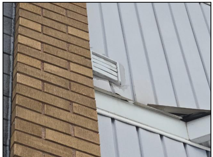
Improper Plastic Vent Termination
