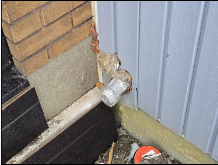
Caulking missing or ineffective
