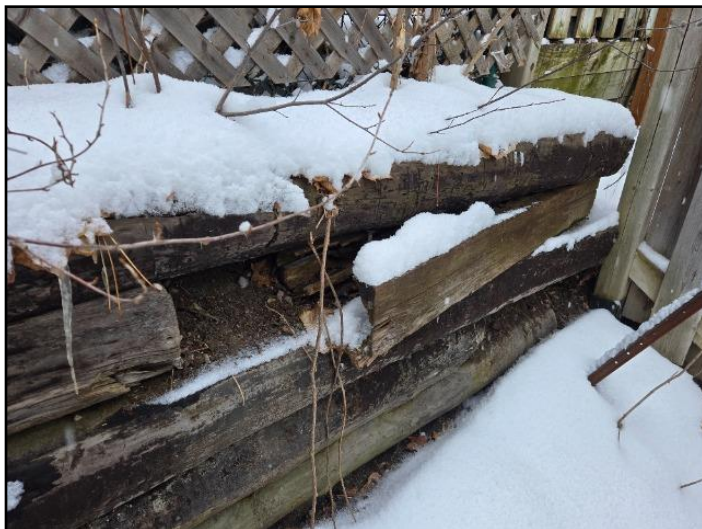
Wall exhibit signs of deterioration
