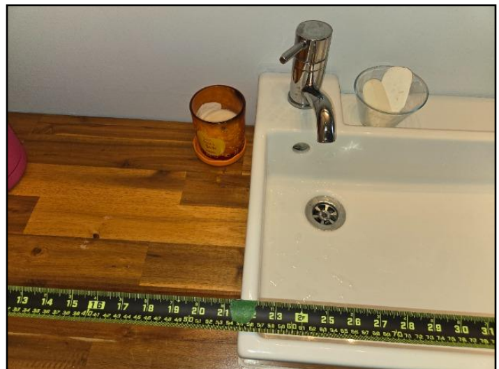
No GFCI/GFI (Ground Fault Circuit...)
