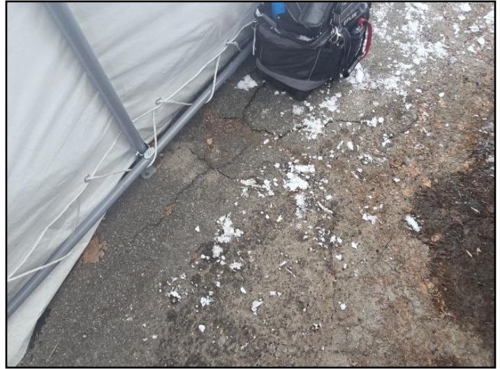
Cracked or damaged surfaces
