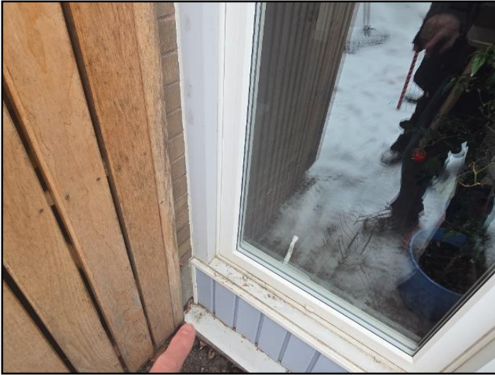
Caulking missing or ineffective
