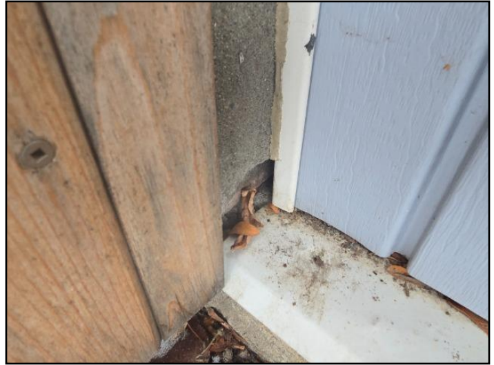
Caulking missing or ineffective
