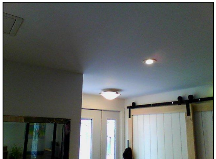
Gaps or voids
