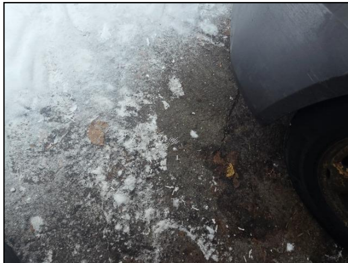
Cracked or damaged surfaces
